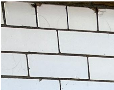
Plate 1: Holed / cracked Ceramic Bricks
