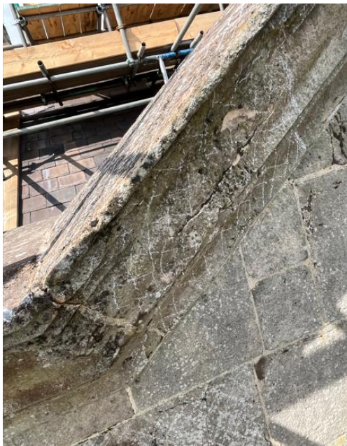
Plate 1: Existing stone face delaminations Marked with chalk and templated for replacement
