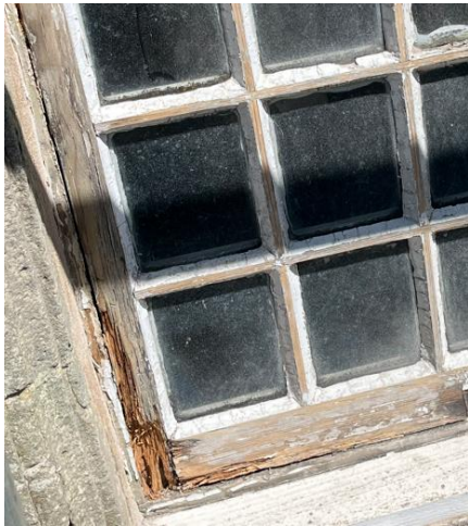
Plate 1: Rotting of existing windows
