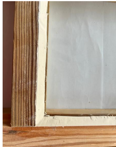
Plate 4: On site fitted and new putties to hold
