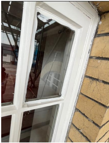
Plate 1: Broken / cracked existing windows
