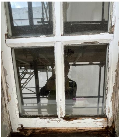
Plate 1: Broken / missing existing putties
