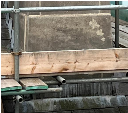
Plate 1: Existing lead flashings
