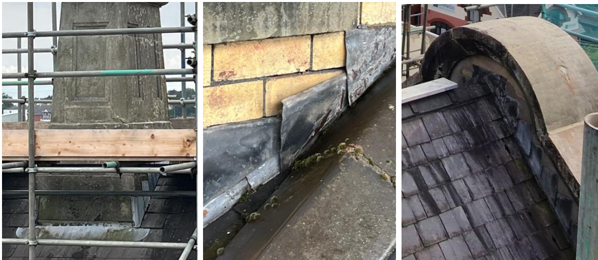
Plates 3,4 & 5: Selection of photographs of defective lead flashings and soakers found existing (code 4 soakers existing, code 6 flashings existing).
