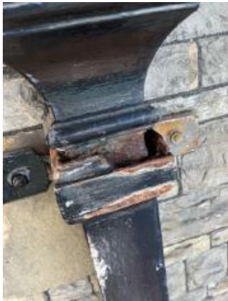
Plate 1: Existing defective rainwater goods
