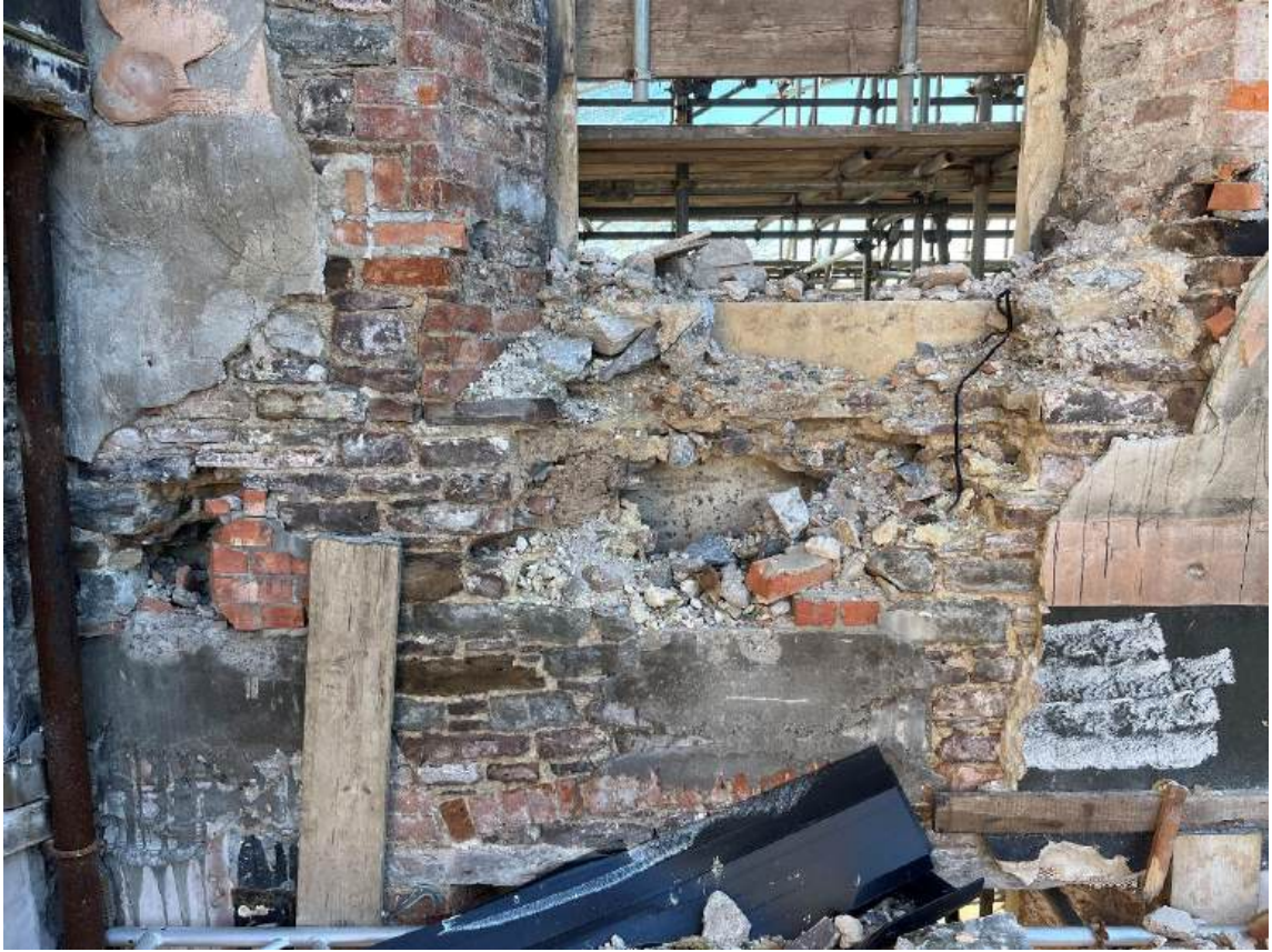
Photo 21 – Showing damaged masonry under the window
