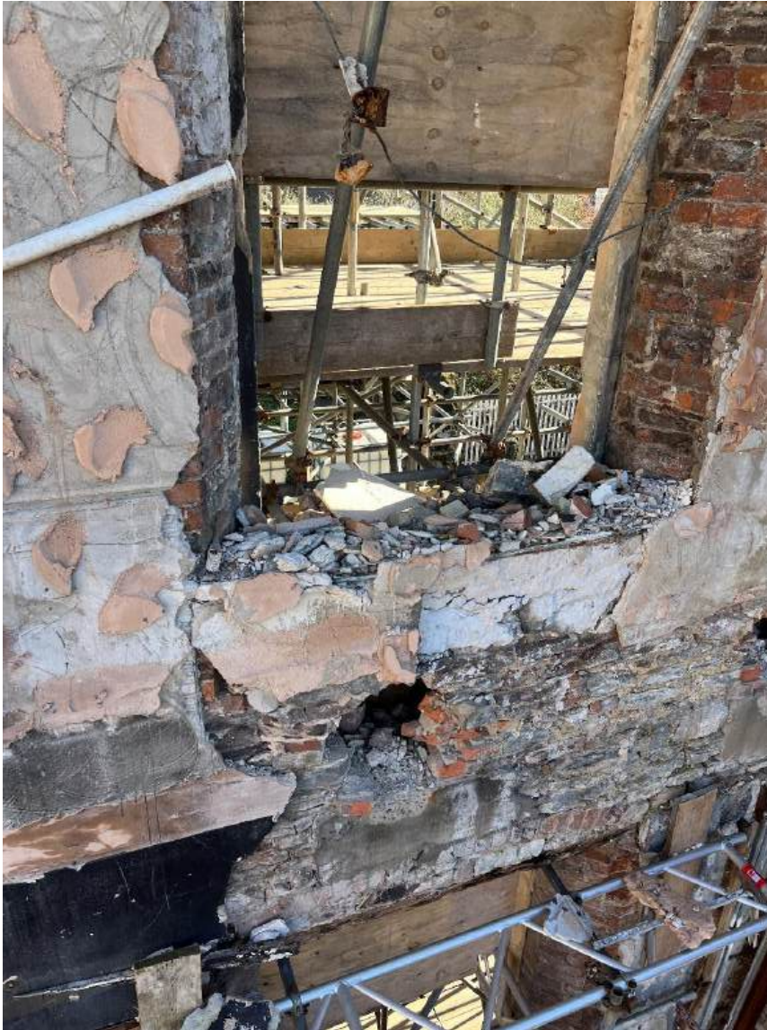
Photo 29 – Showing damaged masonry from steel frame
