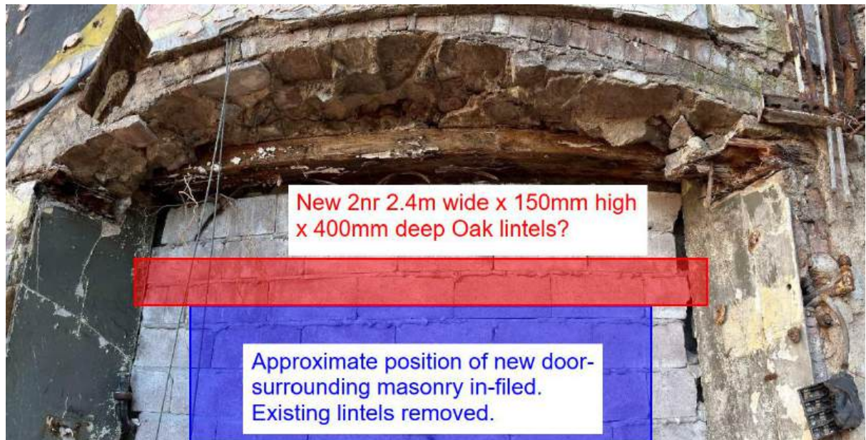
Photo 27 – Showing ground floor window partly blocked up (three photos stitched together)
