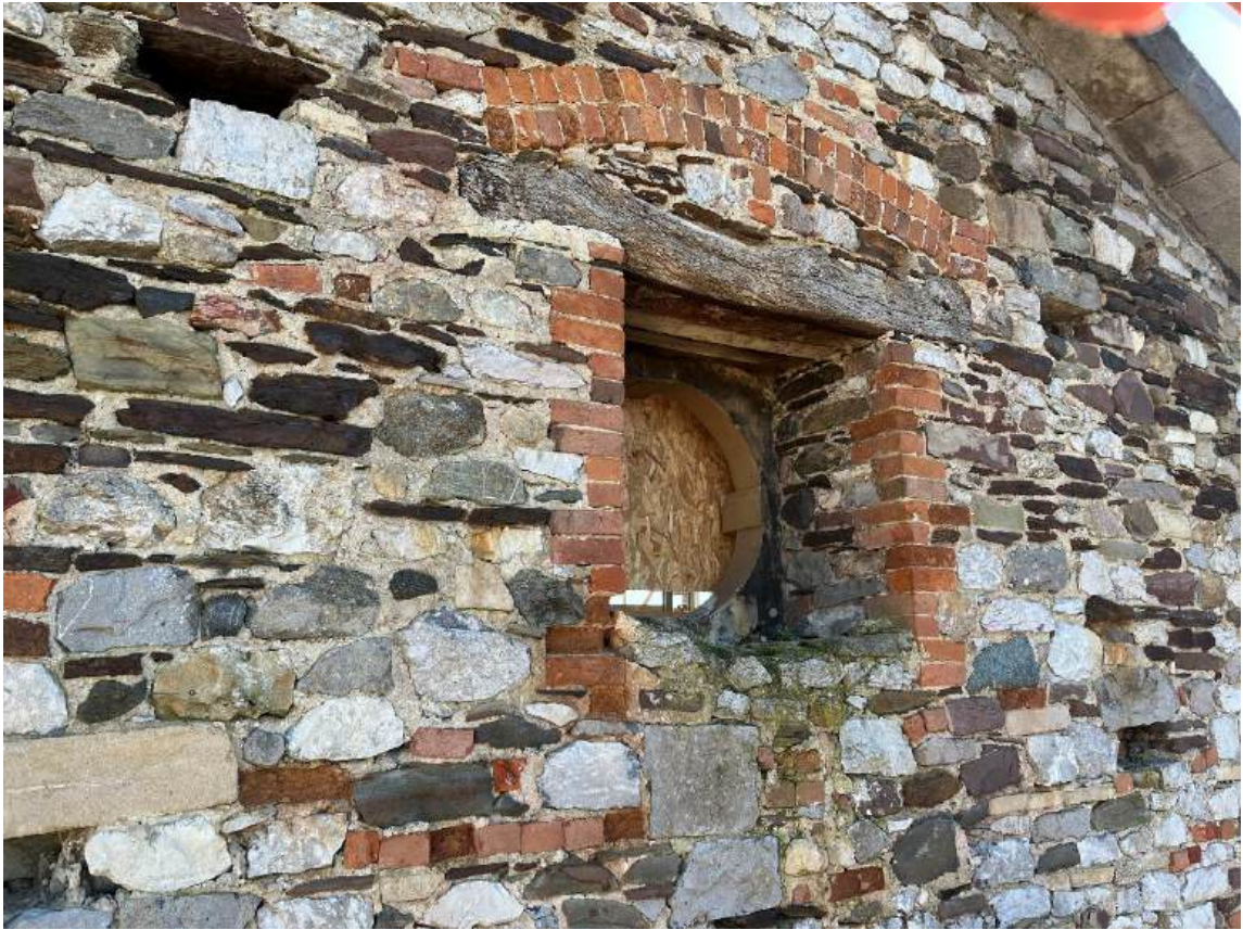
Photo 26 – Showing timber lintel over feature opening in façade
