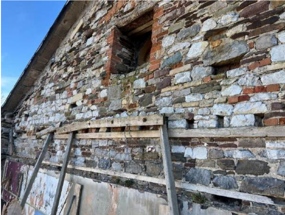
Photo 30 – Showing holes from the built-in timber ceiling joists.
