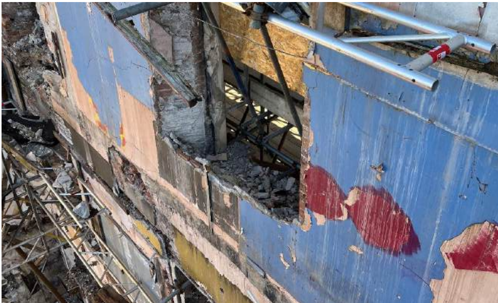
Photo 23 – Showing loose masonry around window cill
