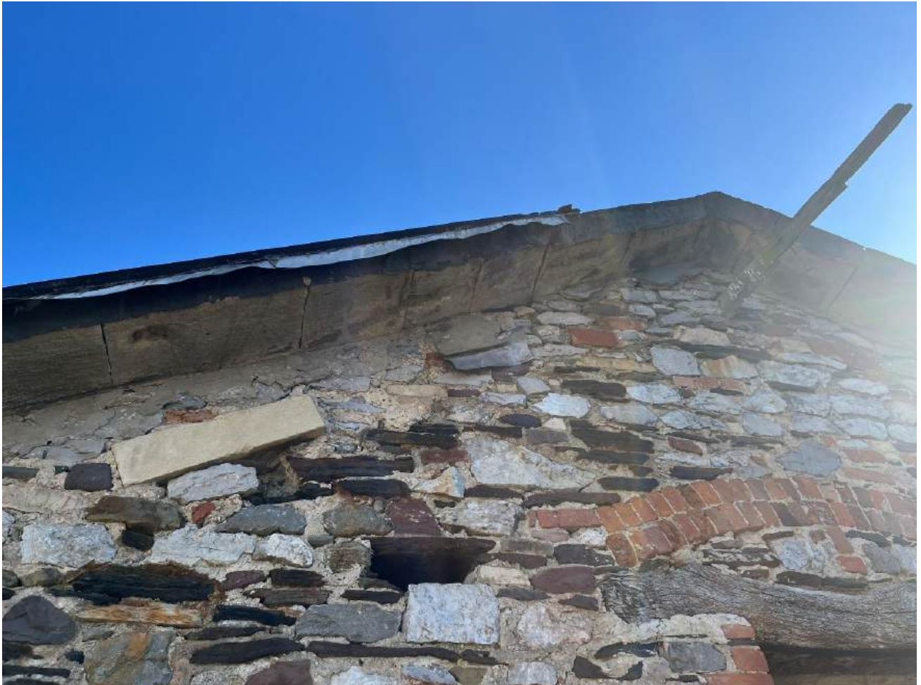
Photo 25 – Showing missing stonework in the façade
