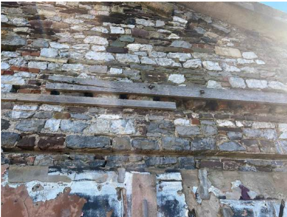
Photo 31 – Showing holes from the built-in timber ceiling joists.
