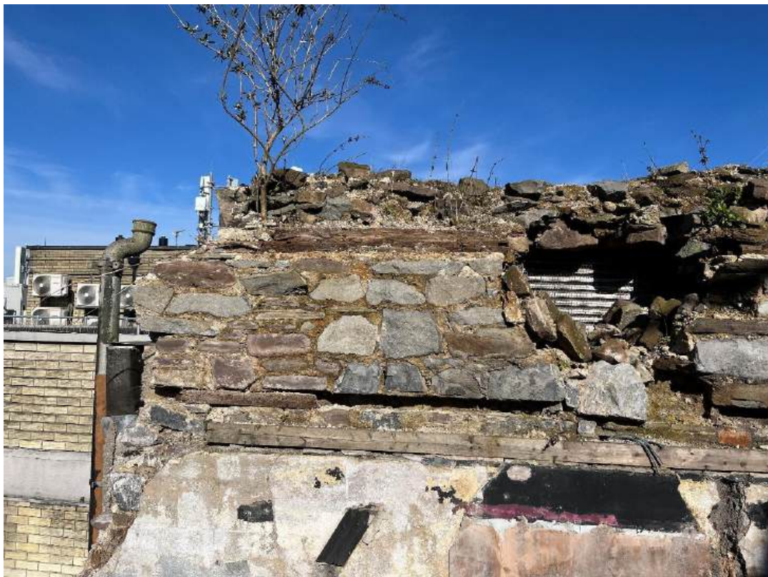
Photo 13 – Showing top of the wall with uneven stonework and vegetation growth
