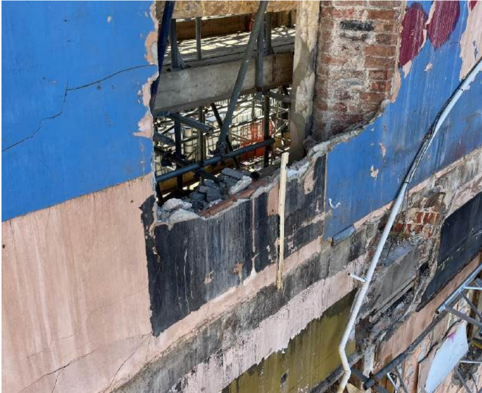
Photo 22 – Showing loose masonry around window cill
