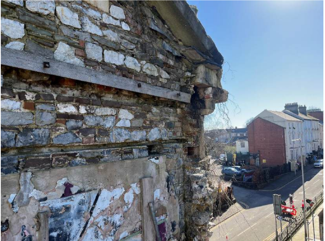
Photo 32 – Showing the remainder of the wall with plant growth
