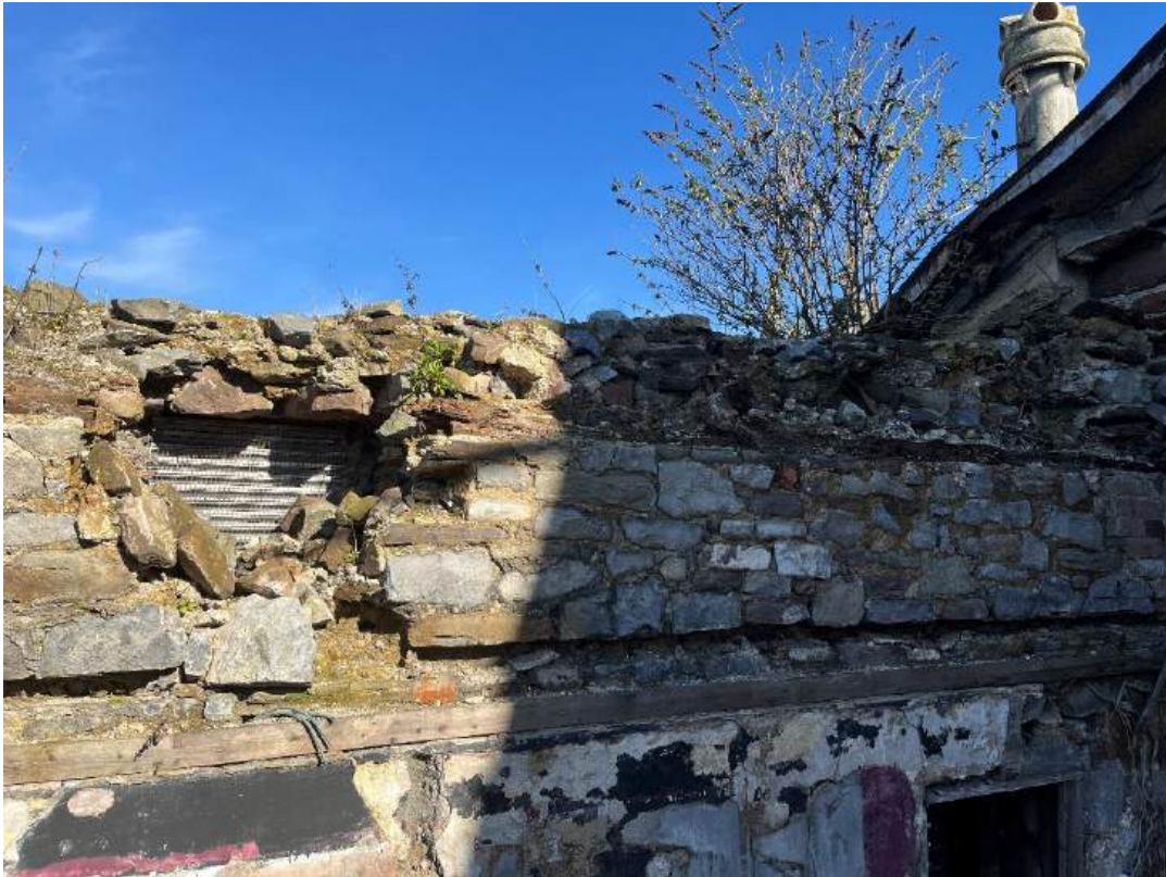
Photo 14 – Showing top of the wall with uneven stonework and vegetation growth
