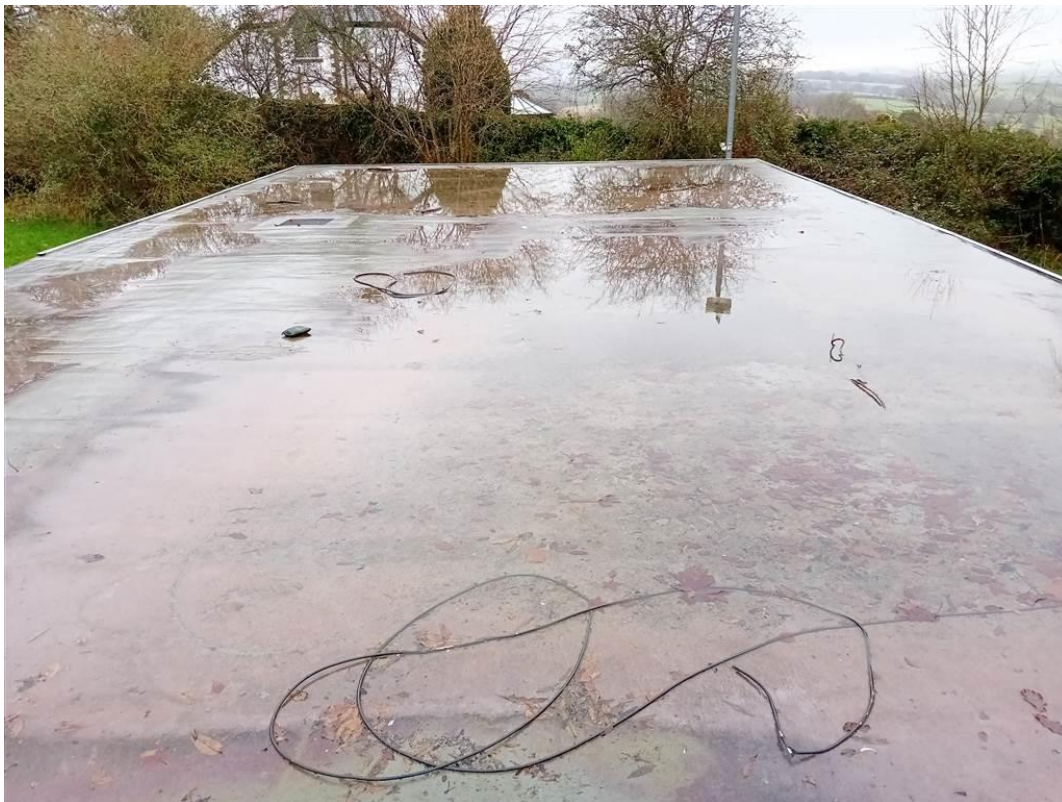
Left: Significant ponding on annexe roof (2024)
