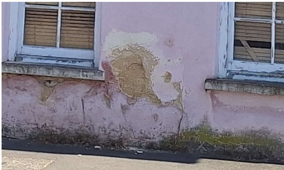
Fig. 1. Defective Render to front Elevation
