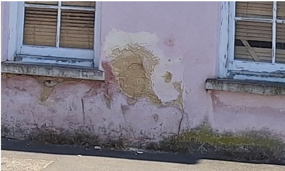
Fig. 1. Defective Render to front Elevation
